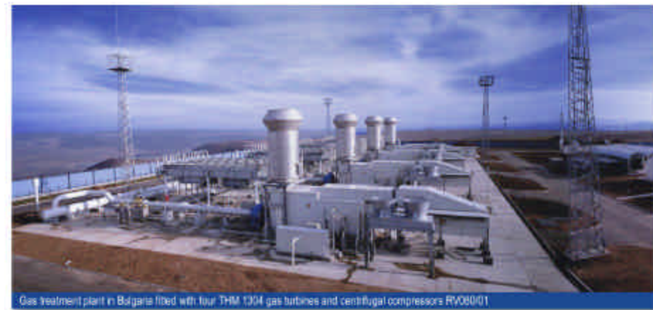
Gas treatment plant in Bulgaria fitted with four THM 1304 gas turbines and centrifugal compressors RV080/01
