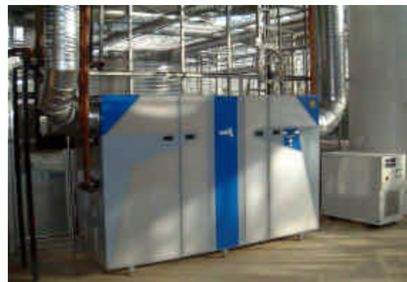
100 kW Turbec microturbine in green house
